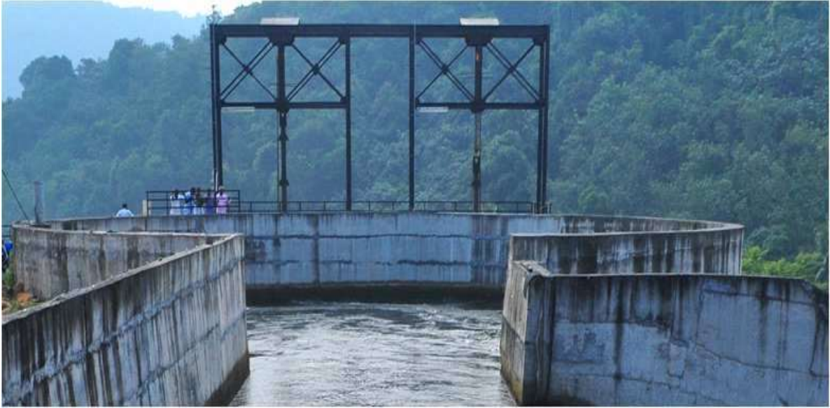
Fig 1.9: Fore bay tank
